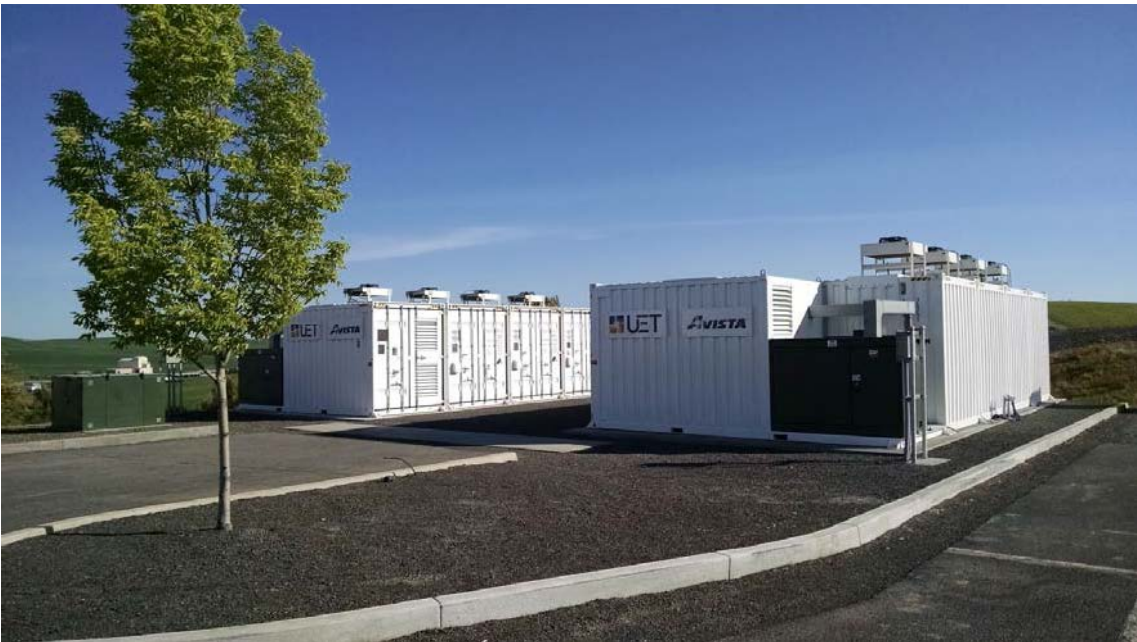
1 MW 4 MWh Turner Energy Storage Project in Pullman from Wikimedia Commons.
