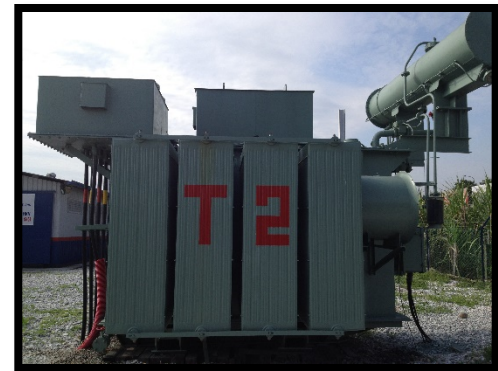
No action taken on the transformer
