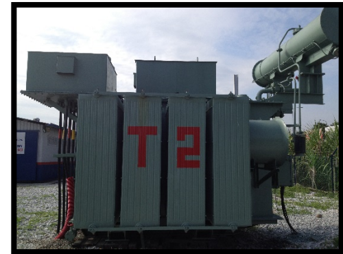
Transformer back into service
