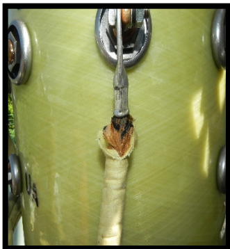
Find the fault location
