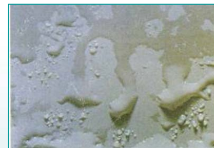
Sand abrasion of insulator skirt
