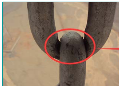
Wear failure of U-rings
