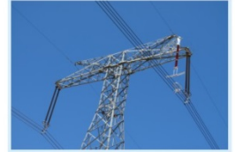
220KV/500KV line arrester
