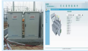
3D-visible operation management platform of transmission line
