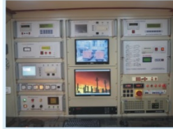
Location metrology vehicles with power Transformer, online inspection vehicle
