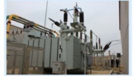
Preassemble Intelligent Substation
