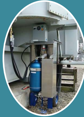
LTC Oil Purification Unit
